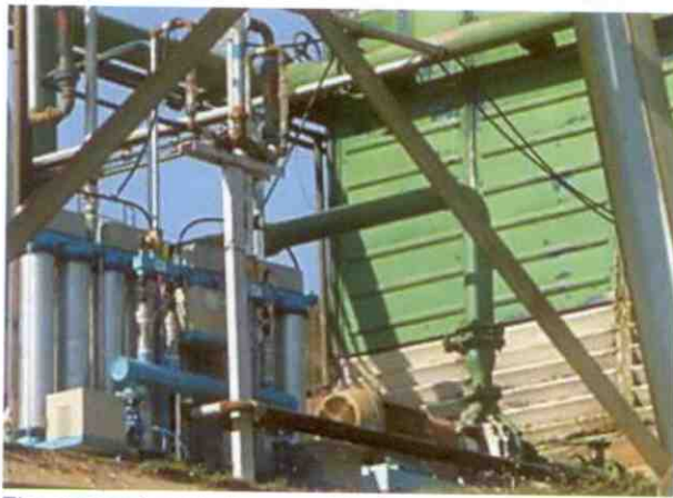
The system installed on a gold mine
